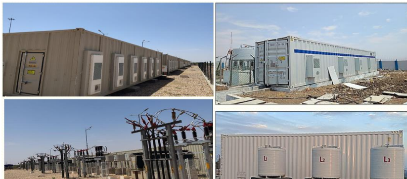
Figure 14: Static VAR generators in solar plant
